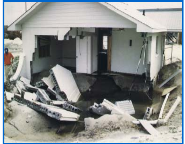
Post-storm field studies have shown that minimally compliant A Zone foundations often fail in Coastal A Zones.
